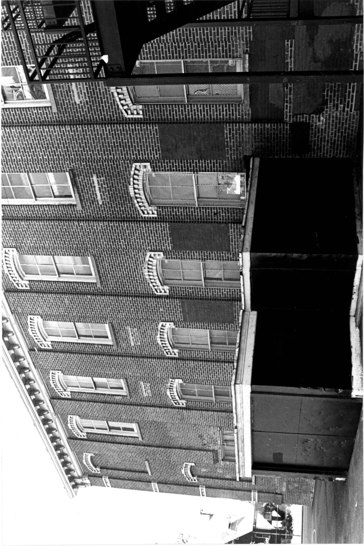
Westfield Township District School No. 5 (now Public School 1 Annex), corner of Yetman Avenue and Academy Avenue, Totterville, Staten Island. North facade, original wing. Photo: Carl Forster
