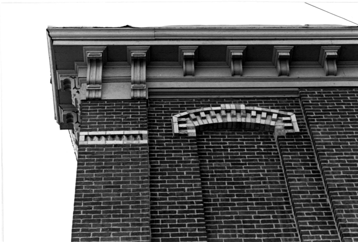
Westfield Township District School No. 5 (now Public School 1 Annex), corner of Yetman Avenue and Academy Avenue, Tottenville, Staten Island. Detail, cornice, original wing.
