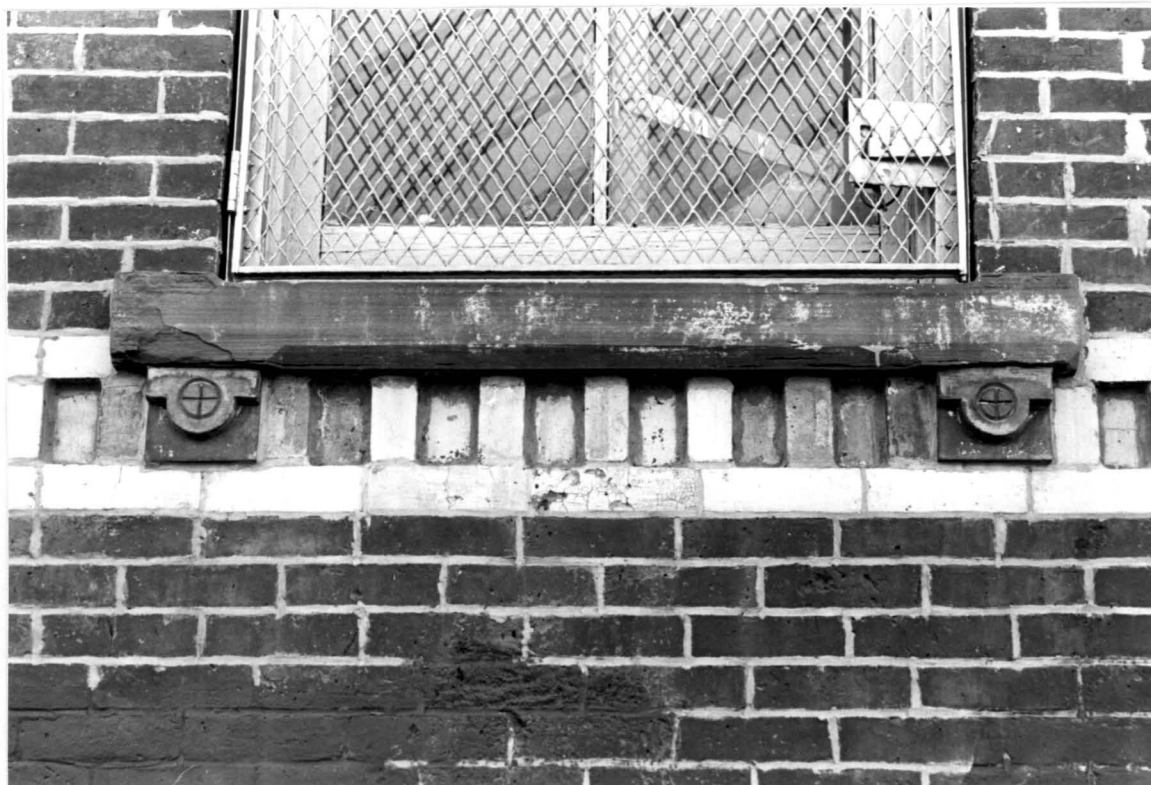
Westfield Township District School No. 5 (now Public School 1 Annex), corner of Yetman Avenue and Academy Avenue, Tottenville, Staten Island. Detail, window sill and decorative banding, original wing.
